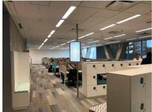
Efficient lighting in the call centre and other rooms with natural daylight due to constant lighting control systems.
