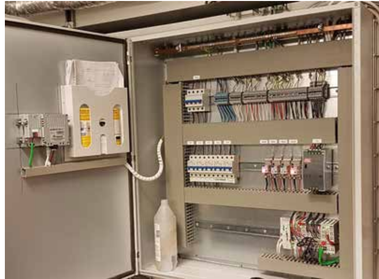
A Wago PLC with a KNX module regulates the hot water outside heating.
