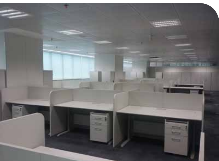
Optimum lighting conditions in the shared offices thanks to the coupling of shading and constant light controllers
