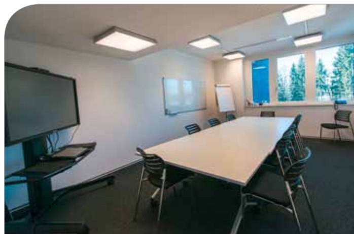
The KNX bus devices control all lights on the 12,400 m 2 – the benefits of DALI lighting control to be used with dimming and lighting control
