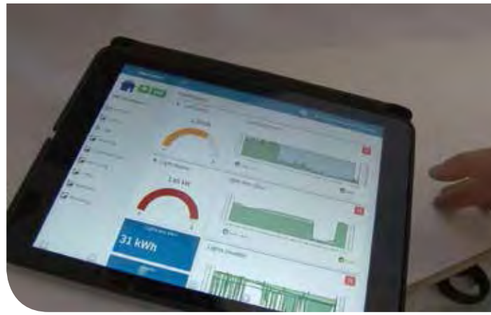
KNX visualisation – RGB White lighting system, Nest climate control system, access control, energy management.
