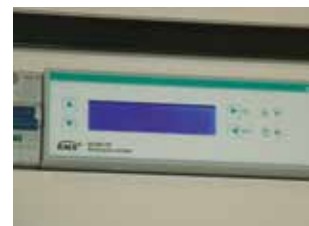
An ekinex® KNX mixing actuator controls the servo motor of a mixing valve delivering the correct temperature to the fan coil circuits
