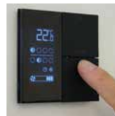
End users can modify the setpoint of \pm 2^{\circ}\text{C} and manually control the fan speed
